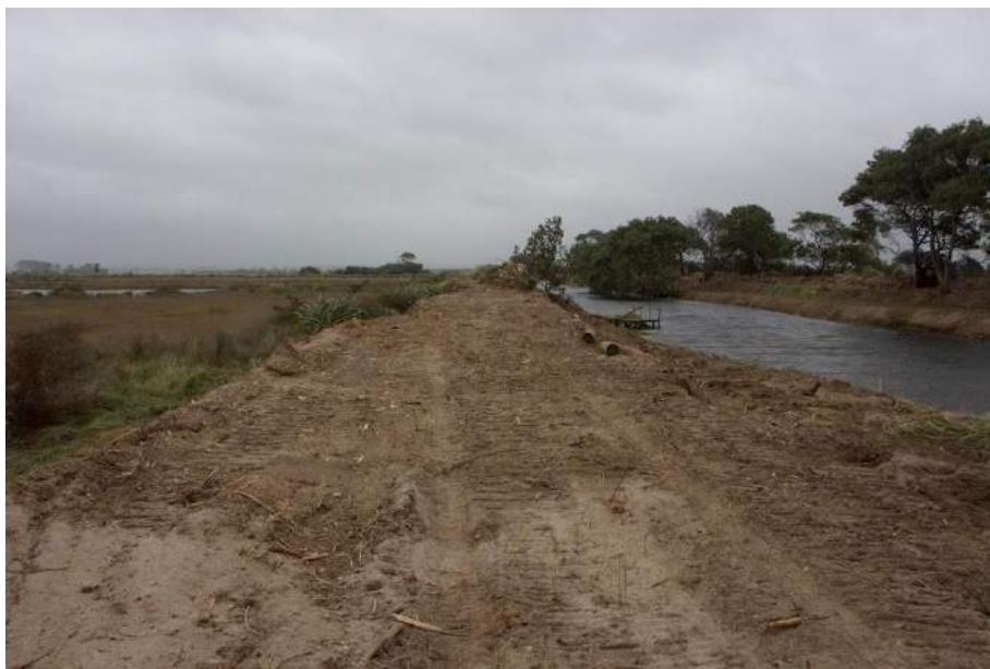
Stopbank on the eastern section of the reserve - looking south up the Pongakawa stream.
